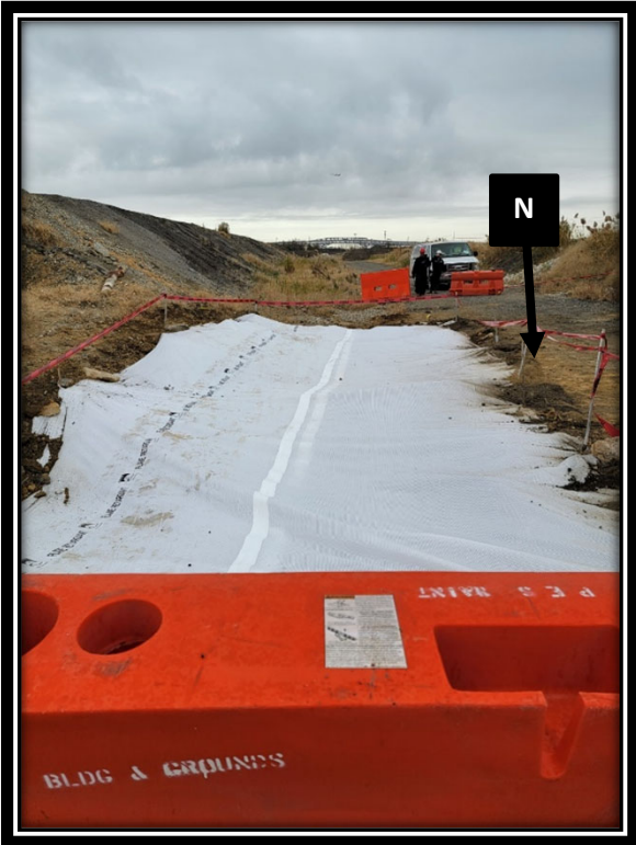
Poly insalled in advance of rain event keyed in and sloped to prevent runoff into excavation
