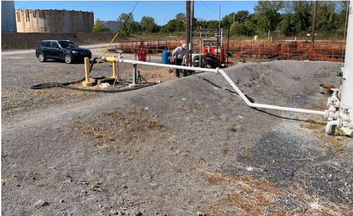
Photo 1: Photograph of flange where staining was noted by tank inspector in March 2022.
