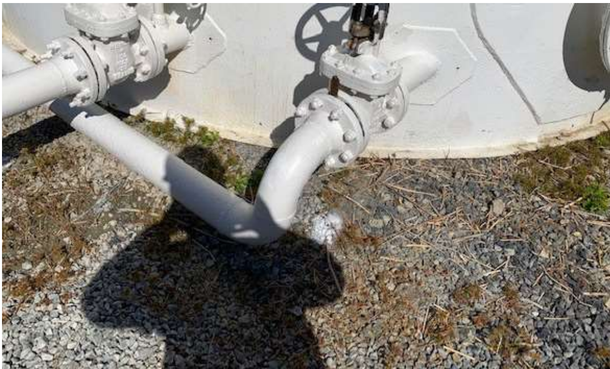
Photo 2: Photograph of flange where tank inspector identified oily residue on exterior of piping in March 2022. No clear staining observed on ground surface and no remaining residue on piping.
