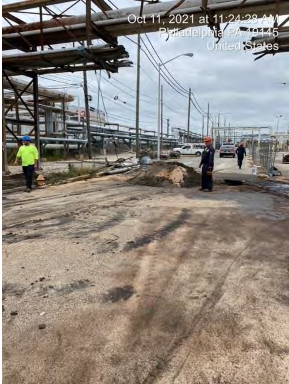
Sorbent material and excavated soil being stockpiled while waiting for a lined roll-off to arrive from the empty container laydown area.
