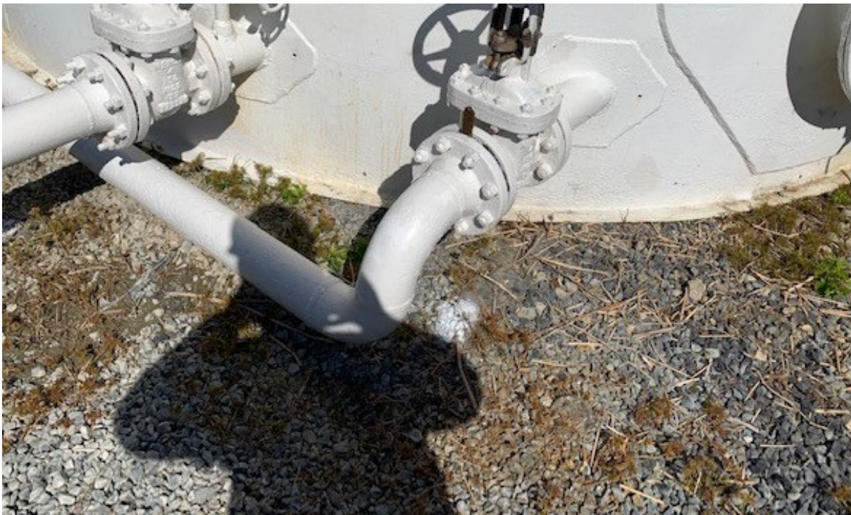
Photo 2 (February 2023): Photograph of flange where tank inspector identified oily residue on exterior of piping in March 2022. No clear staining observed on ground surface and no remaining residue on piping.
