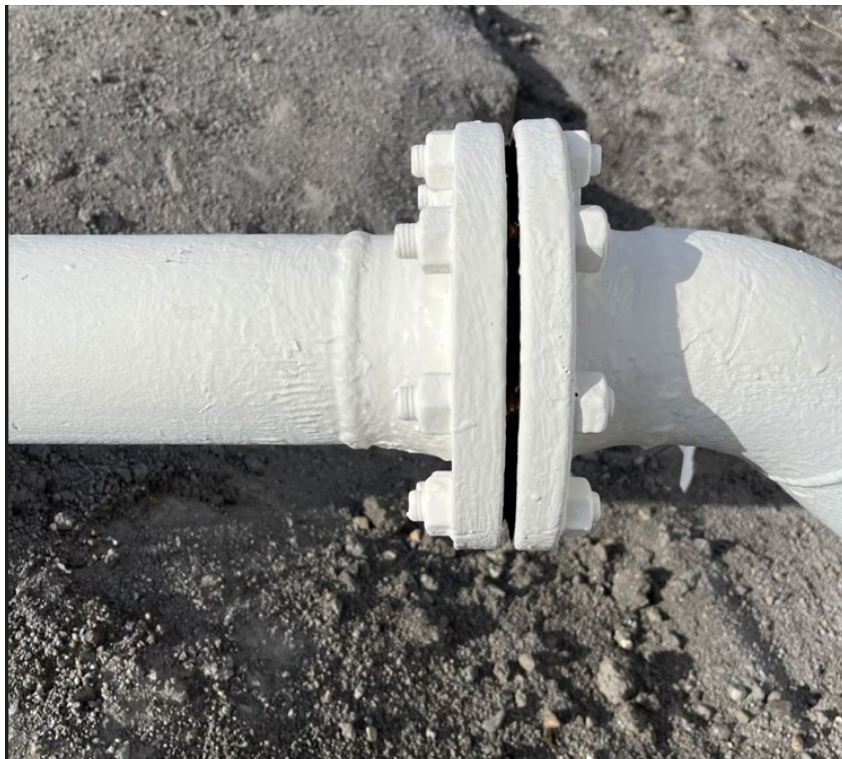
Photo 7 (February 2023): Close-up of the flange previously noted in the inspector report.
