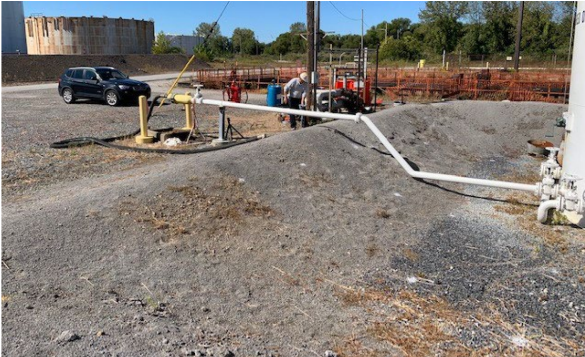
Photo 1 (September 2022): Photograph of flange where staining was noted by tank inspector in March 2022.
