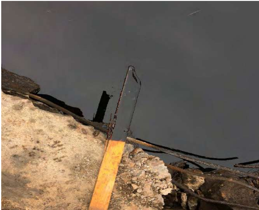
Photograph 4: View of NAPL beneath the tank foundation at Tank 025A (GP R 281).
