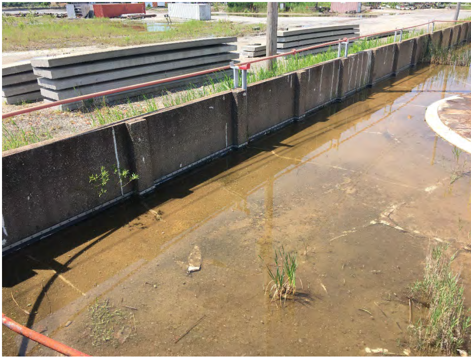
Photograph 6: View of Tanks 1086 and 1087 pad with notable cracking and standing water.
