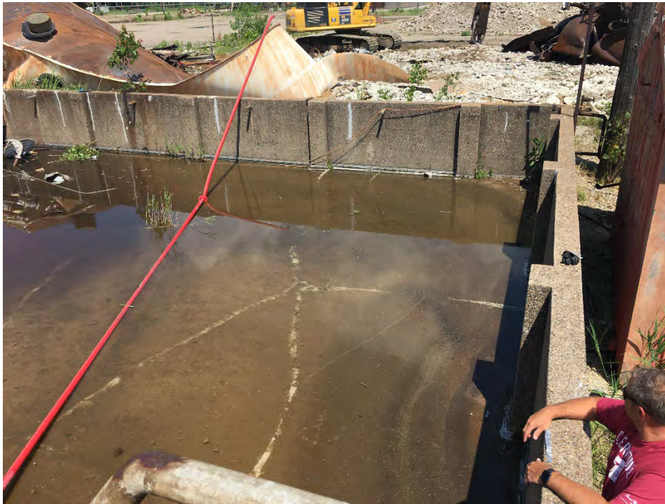
Photograph 7: View of Tanks 1086 and 1087 pad with notable cracking and standing water.
