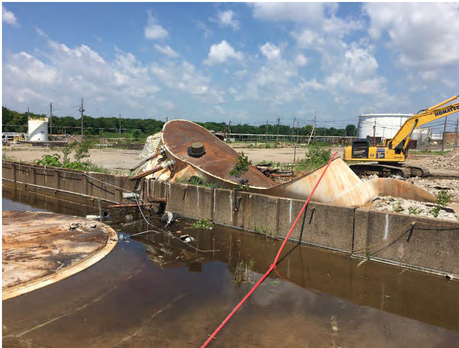
Photograph 8: View of demolished tank outside of pad.
