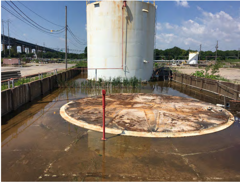
Photograph 5: View of Tanks 1086 and 1087 pad with notable cracking and standing water.
