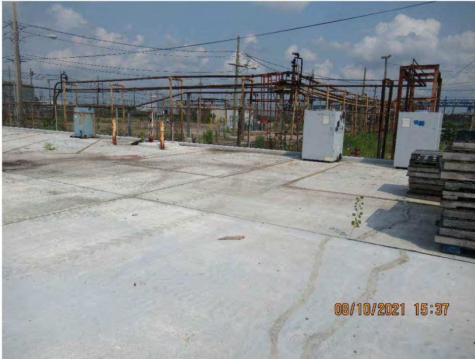
Photograph 3: View of Girard Point Hazardous Waste Storage Pad with notable staining prior to paving.
